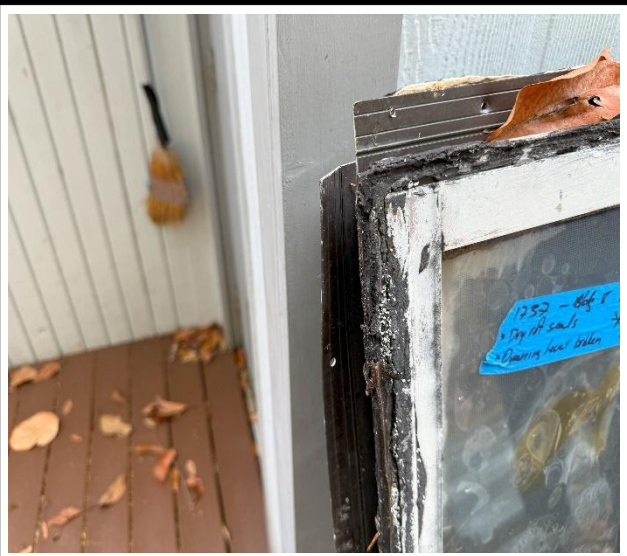
Photo 3 : Bad Window Frame
