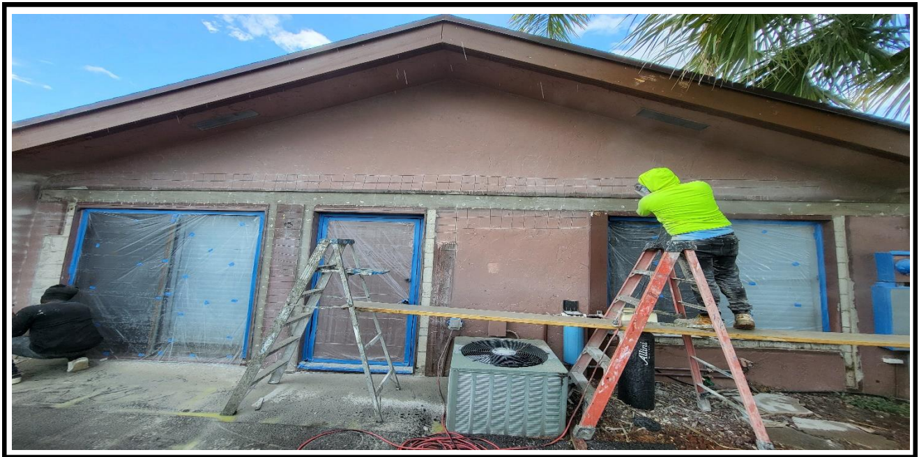
2 – Ongoing, Marking of the delaminated stucco at exterior wall, BLDG 18.
